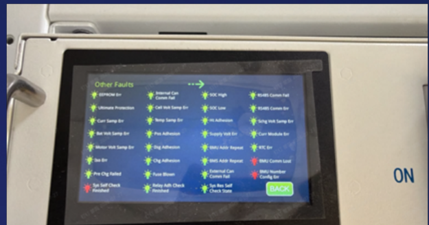
High voltage battery alarm
